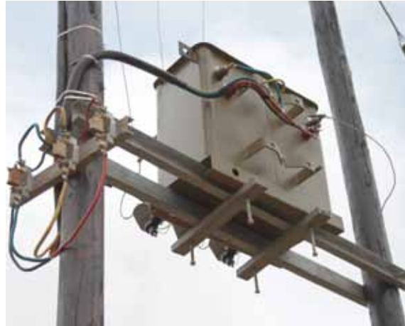
Photograph of a Well-Installed Distribution Transformer
