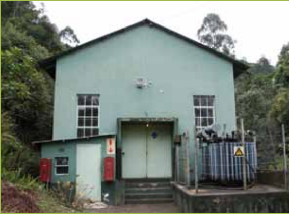
Mbabane Hydro Power Station
