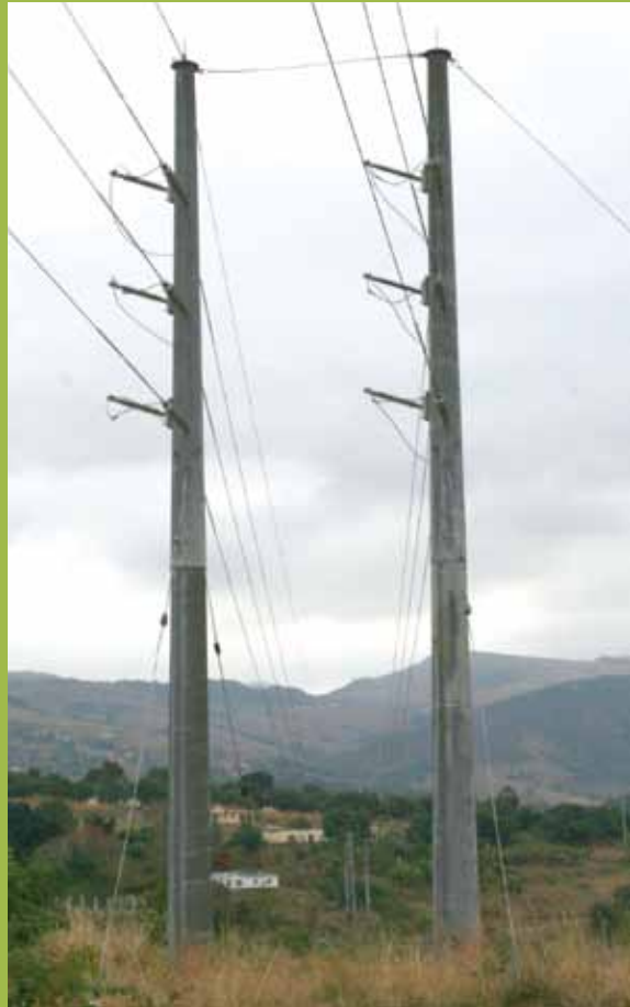
Ezulwini Dual Steel Monopole
